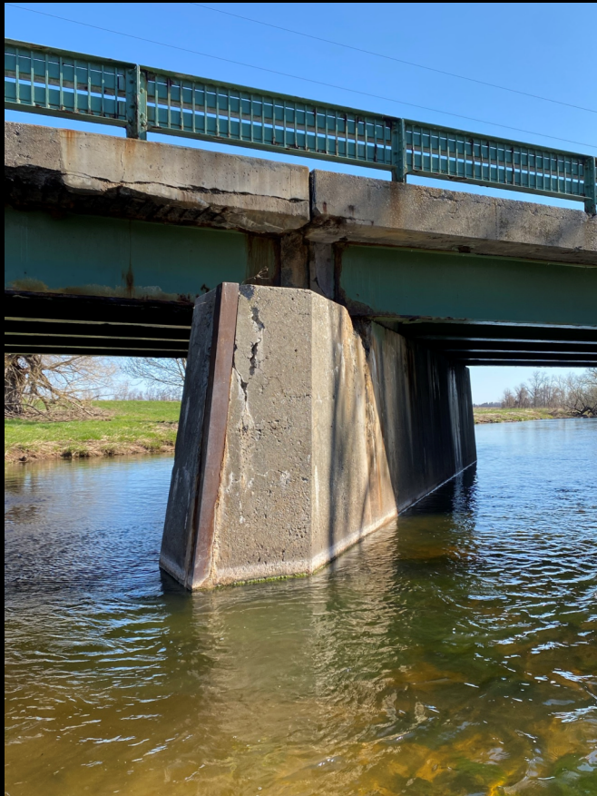
Concrete pier nose condition
