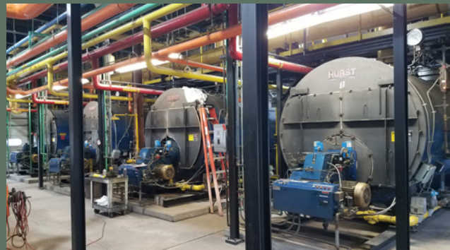
Iola Powerhouse & Cogeneration Facility
