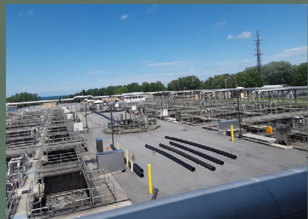
Monroe County Water Resource Recovery Facility
