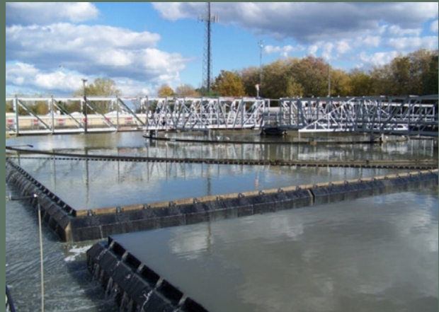
Monroe County Water Resource Recovery Facility
