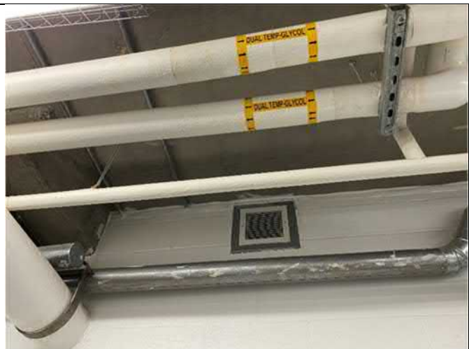
Dual Temp Glycol Piping
